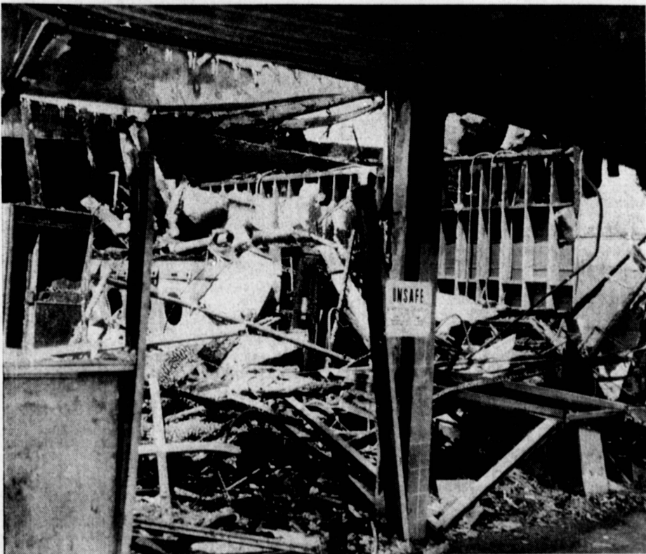
AFTERMATH OF FIRE . . . More than $100,000 in damages was reported here Thursday after flames swept through stores in the Carson Shopping Plaza at Carson Street and Normandie Avenue. The flames broke out in a laundry and spread to three
