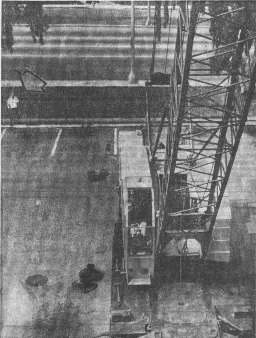
UP WE GO — This overhead view, swinging from the top of the crane at left, was taken by The Press' young summer photographer, Mitch Major. Man on the ground at right, Dick Emery, photographer for another newspaper, stayed on ground at Torrance City Hall, watching, as Mitch went soaring above city hall roof to take photograph below.
