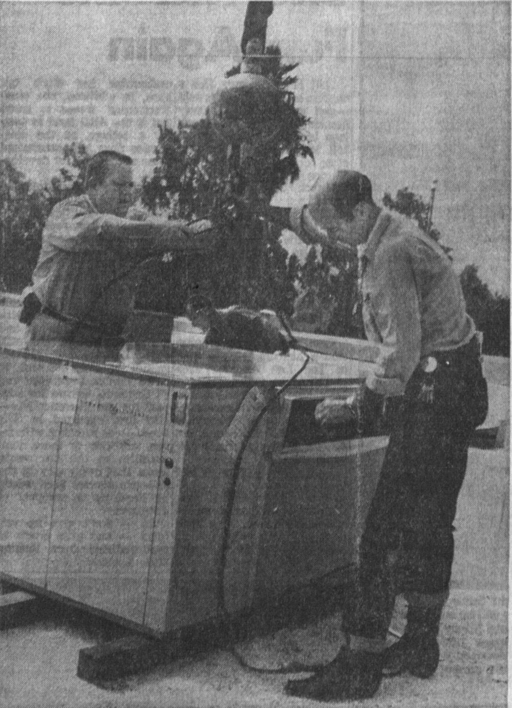
AIR CONDITIONER is eased down the roof of Torrance City Hall by two workmen. The $5186 unit was installed this week in the council chambers, where sweltering heat and large crowds have made transaction of city business uncomfortable. (At least, that's what we were told was the trouble.)
