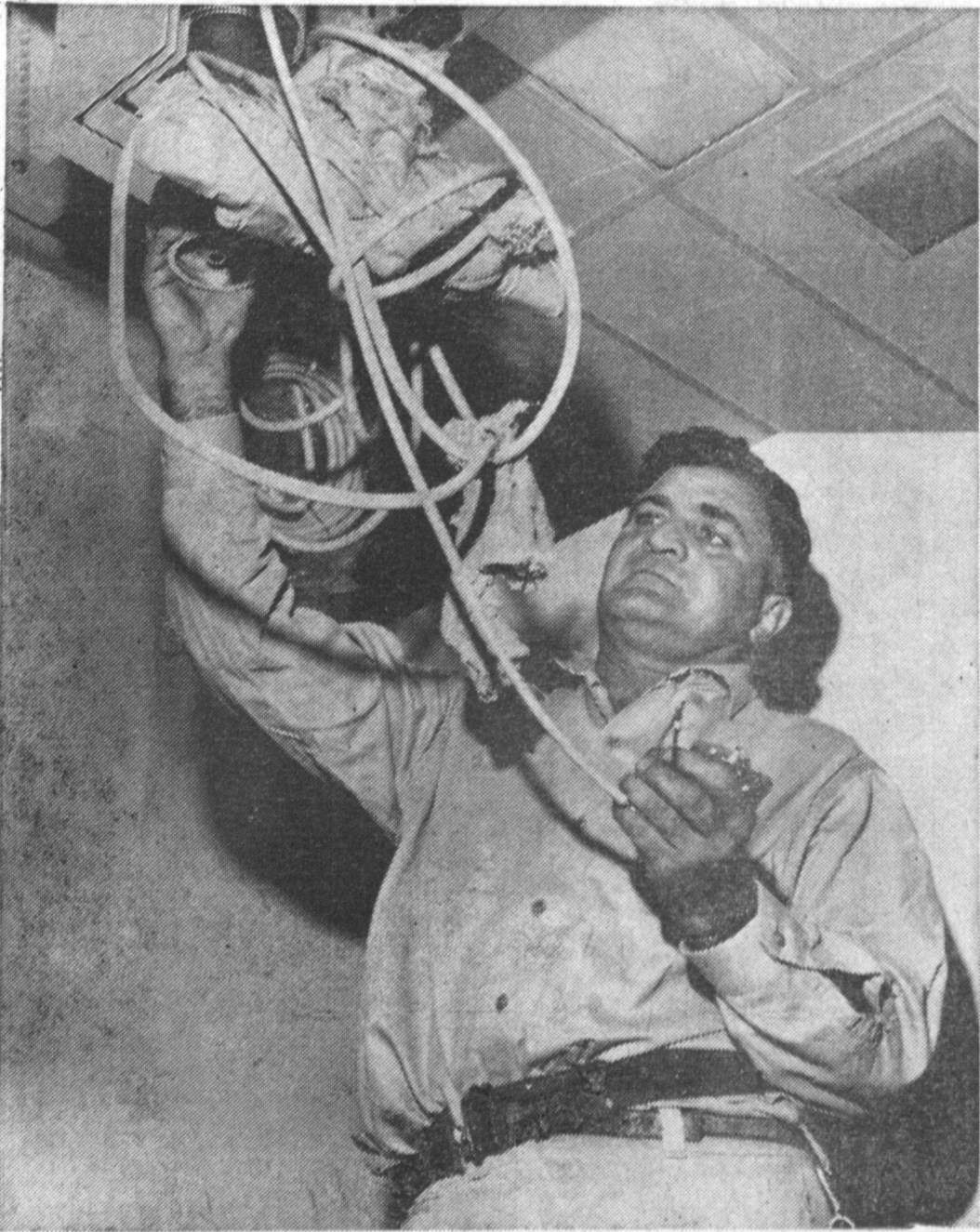
MAZE OF WIRES are sorted out by county electrician Harry Harrison, as one of the many new X-ray machines at Harbor General Hospital is installed. Each X-ray room in the new hos-
