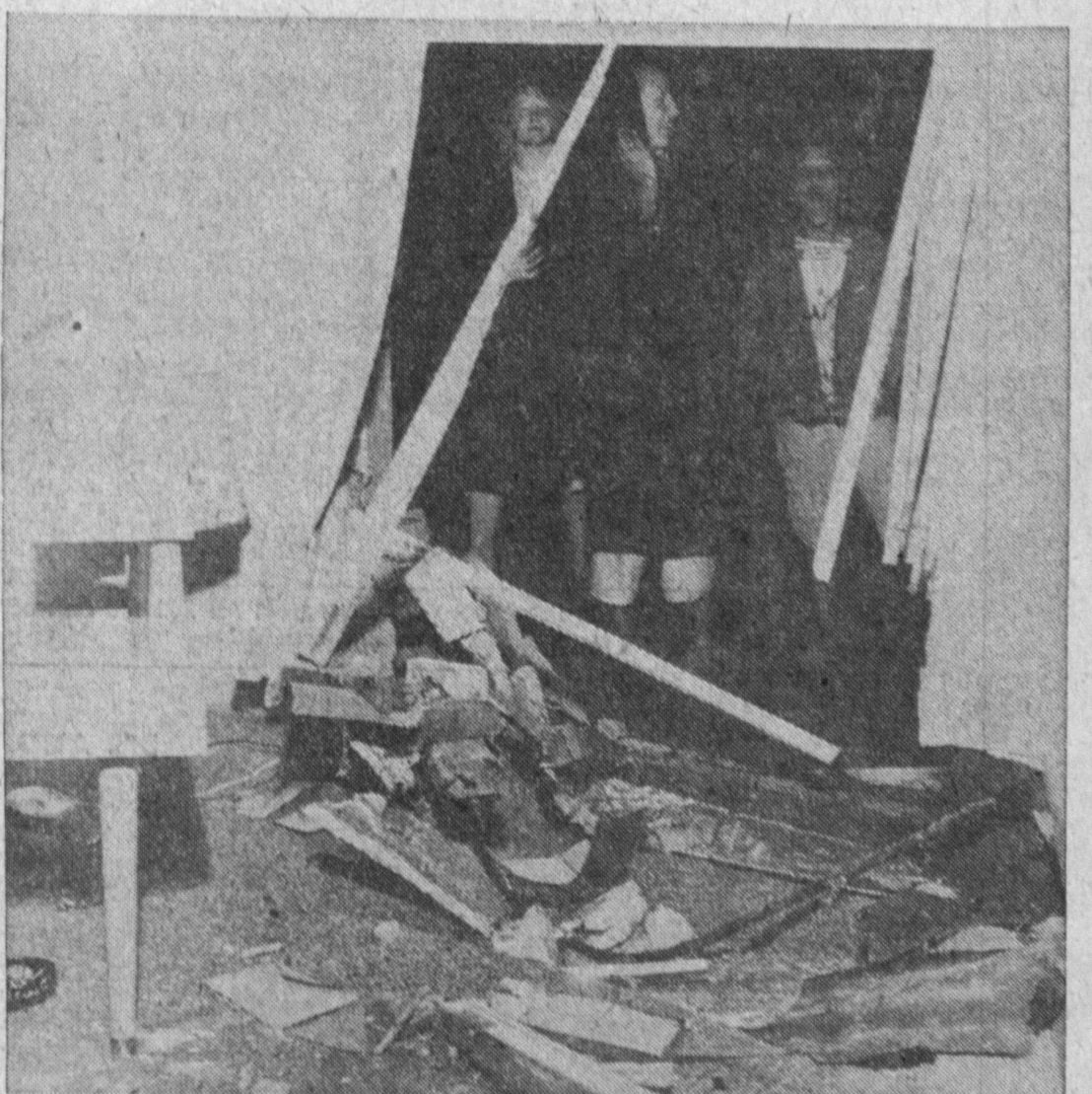
NEW DOORWAY—Torrance homeowner P. J. Chateler of 3403 W. 190th St. found himself the possessor of a new doorway into his front room early Monday morning when a car driven by Jay R. Roysdon, 21, of Redondo Beach went out of control and crashed
