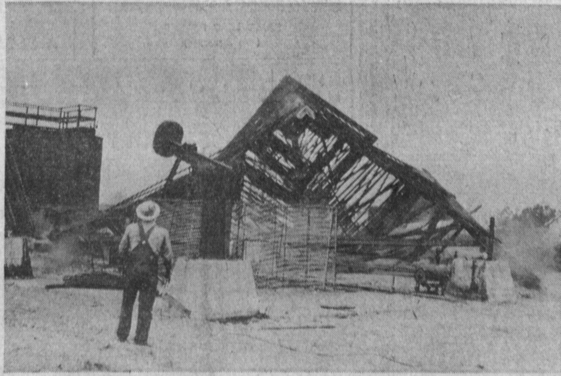
GOING—Tower on 236th St. east of Arlington topples. Planning Director George Powell all had highest praise for oilmen's cooperation. All fields must be cleaned up by 1961.
