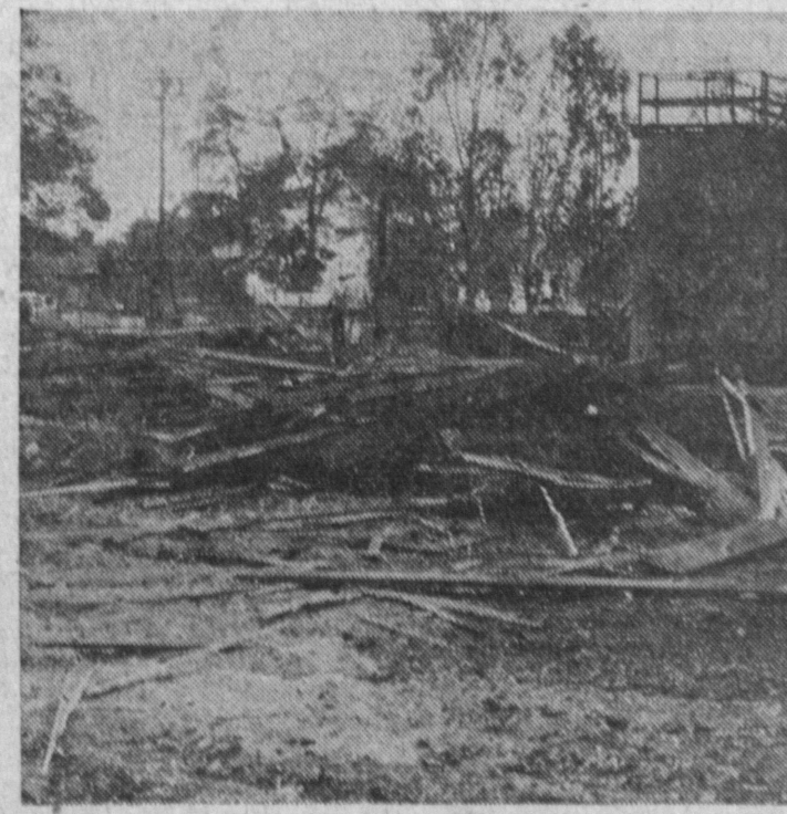
GONE—Only a few men still know how to throw a derrick. Powell appreciates demolition now, rather than at 1961 deadline. —Press Photo
