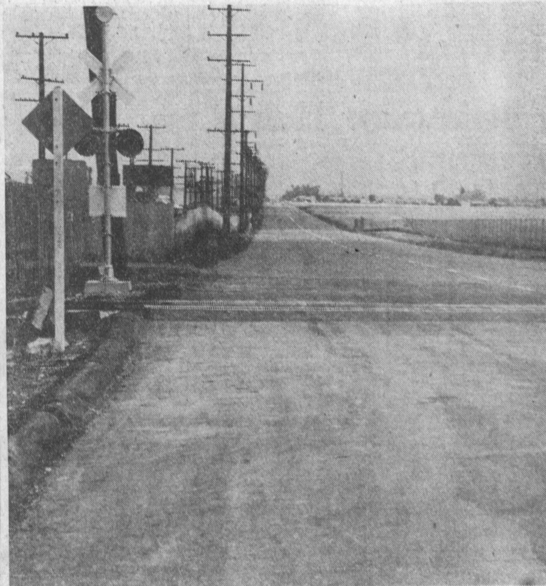
CONTROVERSIAL ROAD —This section of Arlington Ave., which started a probe of public works projects, was finally opened to Del Amo Blvd. Thursday. Crumbling surface of street, which was completed only 17 months ago at cost of $90,000, started investigation. Until this week, the road led "nowhere."
