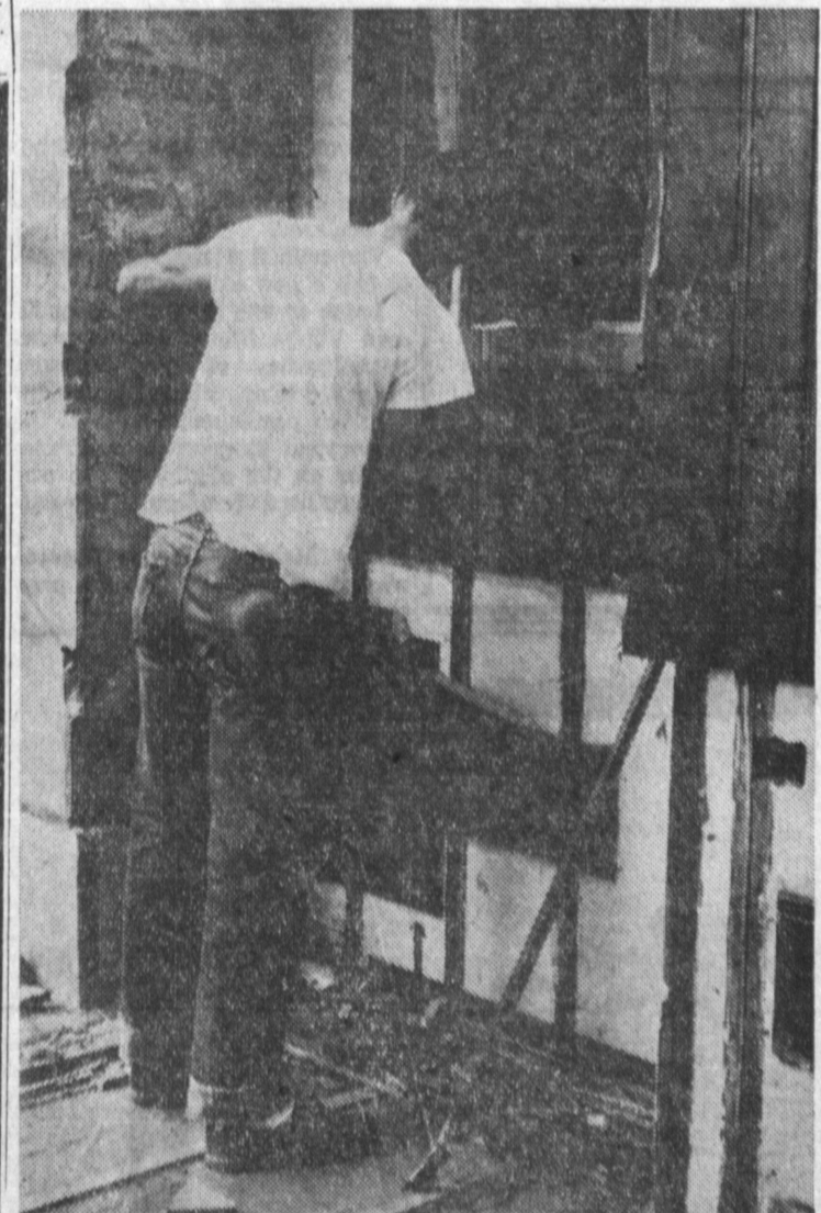
BEGINNING OF END — Lowell Summerford of McAmis and Baker Construction Co., starts work on razing the Carson home on Normandie Ave., north of Carson St., to make room for a new subdivision. The home of Victor Carson, Dominguez Estates Co. official, was built more than 65 years ago and is one of oldest in Torrance. — Press Photo
