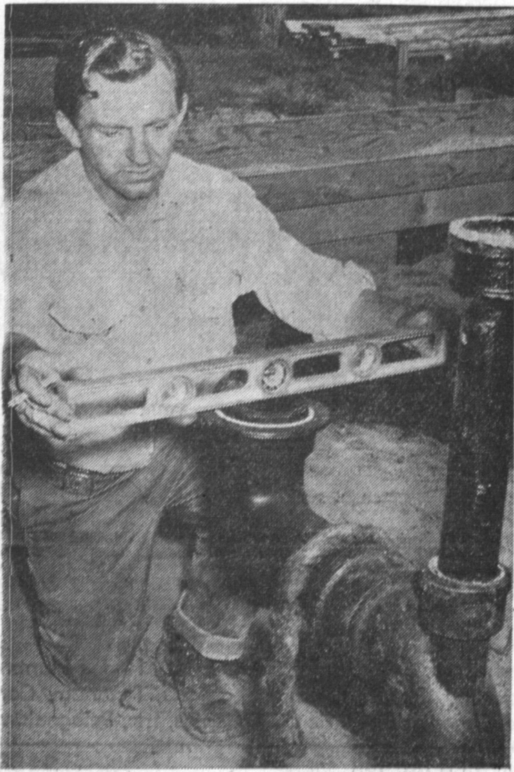
ON THE LEVEL—R. D. Pryor checks the plumbing at the new Torrance Scout Center on Plaza del Amo with a level. Organizations and individuals are donating labor and material for the construction of the building. Press Photo.
