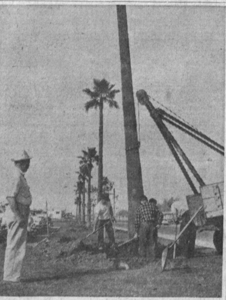
SEVEN-UP —Howard Webb, leadman of this city maintenance crew, looks down the row of newly transplanted palm trees as the other workmen add the finishing touches. The seven trees, which were planted on the city hall grounds at the corner of Torrance Blvd. and Maple St., came from the old Dominguez office on Henrietta St. —Press Photo
