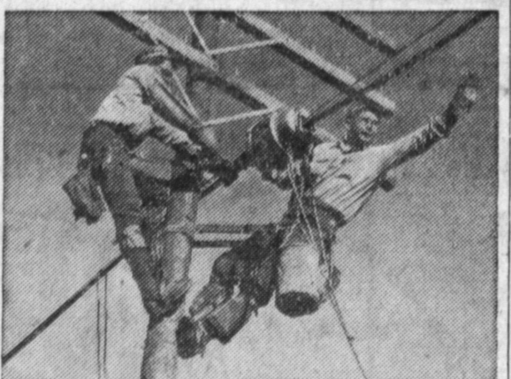
No one can guess the importance of the calls which will flow through the cable these linemen are installing.
