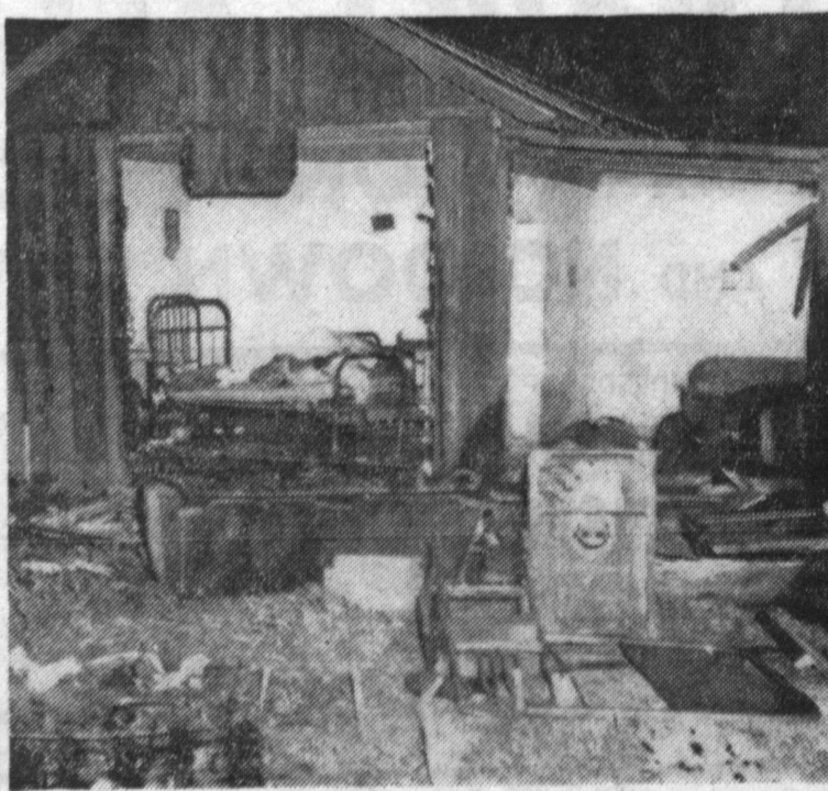
A MATCH accidentally lit in a room filled with butane gas leaking from a small wall heater caused an explosion which tore one wall off home located at 1840 W. 178th St. Owner of the house, Pedro Jimenez, was rushed to the hospital with second degree burns of the hands and face, after the explosion occurred last Wednesday night.
