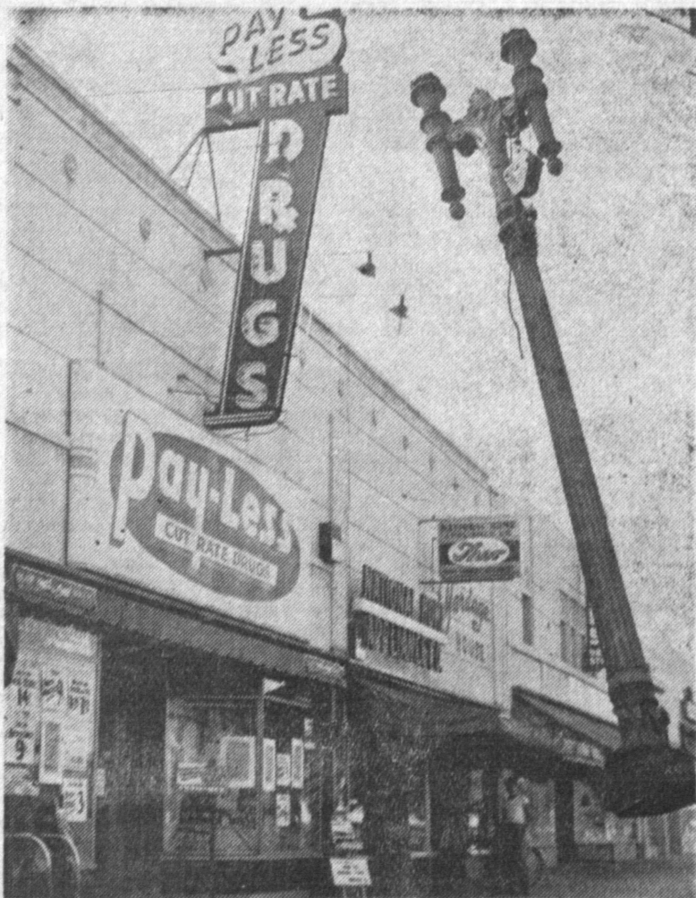
THERE SHE GOES!—Being rooted out to make place for new modern mercury vapor luminous street light in front of Payless Drug Co. on Sartori avenue in downtown Torrance is this old conventional type light standard. The first of the new lights will be installed today. —Press Photo.
