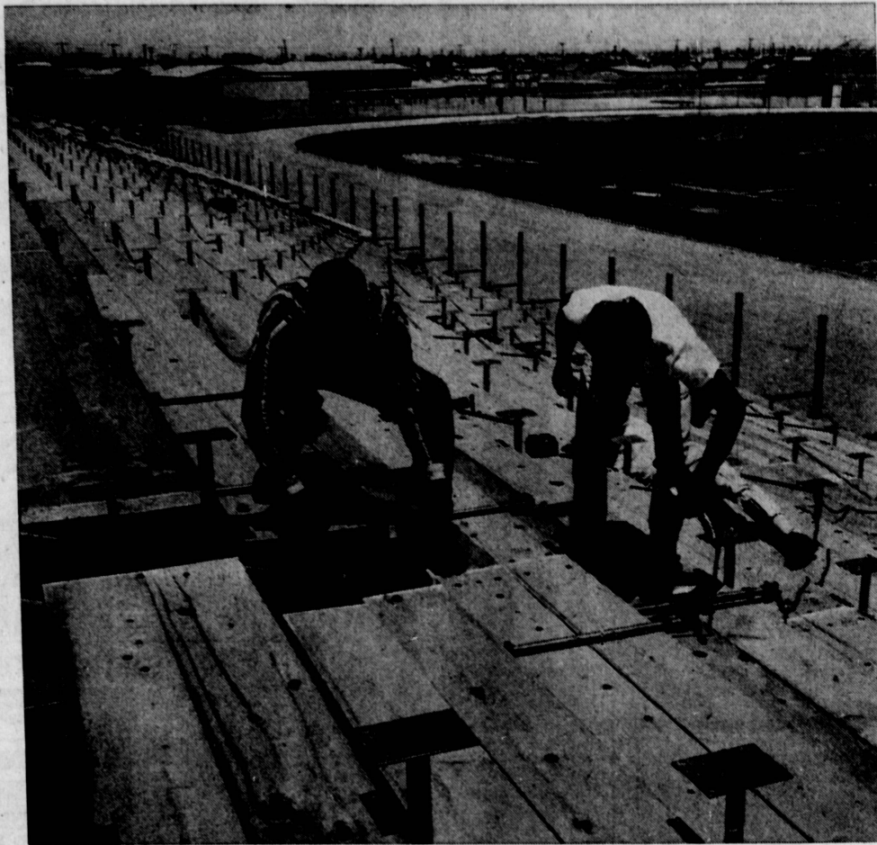
FINAL TOUCHES... Workmen apply the finishing touches to the west-end bleacher section of South High's new $96,000 athletic stadium. The stadium, which housed over 1,000 for Thursday's graduation exercises, is now completed except for bleachers on the east side. Completion of
