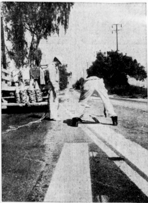
PREPARE INTERSECTION . . . City employees paint white lines which will channel traffic into a right turn lane on Madrona Avenue at Sepulveda Boulevard where traffic signals have been installed. The signals will not be put into service until railroad grade crossing signals are installed. (Herald Photo)
