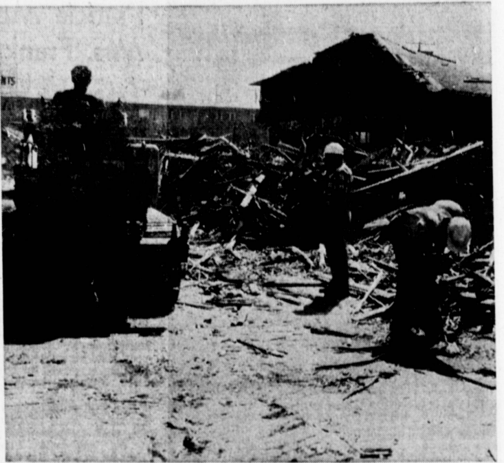
LANDMARK GOES . . . A bulldozer erases a landmark of many years on Pacific Coast Highway as buildings once housing Smith Bros. Fish Shanty restaurant and the Palos Verdes Begonia Farm are leveled to make way for new construction. Evelyn Smith, president of the Smith Bros. Fish Shanty, Inc., said a new two-story building and several shops will be erected at the site. (Herald Photo)
