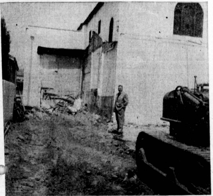
CHURCH EXPANDING . . . The Rev. Hugh R. Percy, rector of St. Andrew's Episcopal Church, checks as workmen near end of demolition work on old sacristy on the church at 1432 Engraecia to make way for $40,000 expansion program. The church will add a Sunday school classroom wing, new sacristy and vestry, and rearrange church seating with the project. (Herald Photo)
