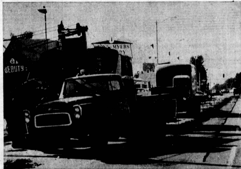
DRAIN STARTED . . . Construction crews for the County Flood Control District have begun work on installation of a new storm drain system to clear storm waters from the area of Torrance Boulevard and Madrid Avenue. Catch basin installations have been made on several Torrance Boulevard intersections and installation of the main line is now ready to start. (Herald Photo)
