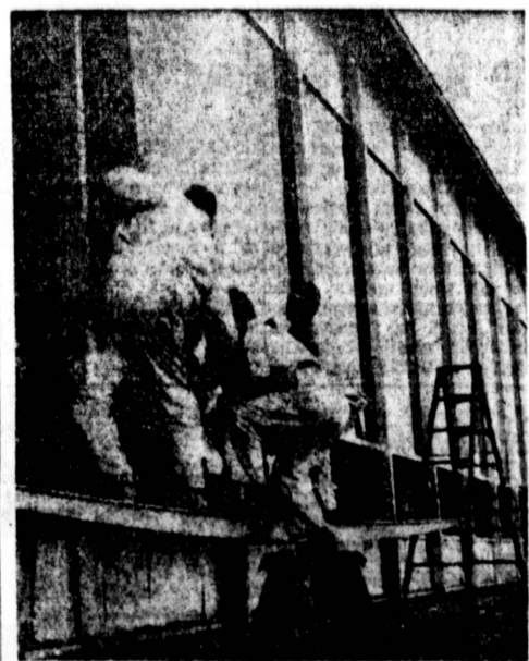
NEARS COMPLETION . . . Workmen place glass in the multi-windowed new Pacific Telephone building at 2154 Torrance Blvd. The two-story structure which will house a "113" information center and the local business office is scheduled to be completed in January.
