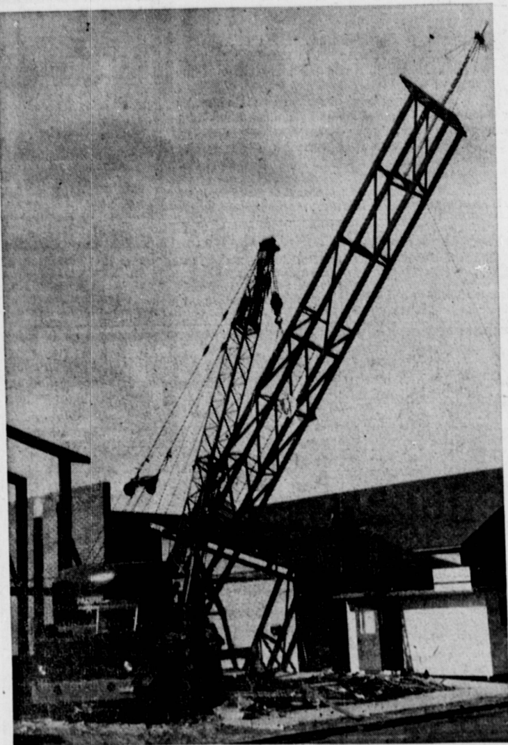
BIRTH OF A LANDMARK . . . Rigging crews and cranes place new bell tower in position where it will dominate the expanded First Methodist Church of Torrance at El Prado and Manuel. When completed, the structure will comprise the new nave and sanctuary for the church. (Herald Photo by Bob Wilton)
