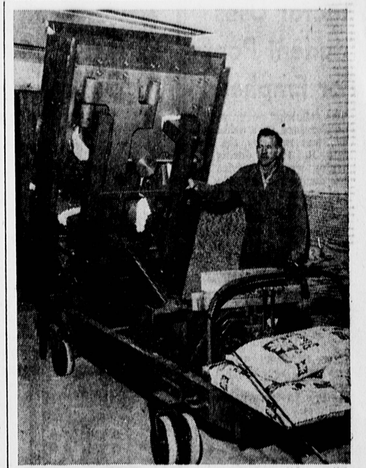
WITHOUT A HITCH!... Four-ton vault door slides easily into place at Bank of America's new Sepulveda and Hawthorne branch, as Alex Bates demonstrates the ease with which his new invention does the job. Bates, vault expert at the bank, worked nearly three years perfecting the hydraulic ram vault door erector, which saves time and avoid installation accidents. The $297,000 bank building at the intersection of Sepulveda and Hawthorne boulevards is scheduled for completion this month. It is near the Broadway department store.
