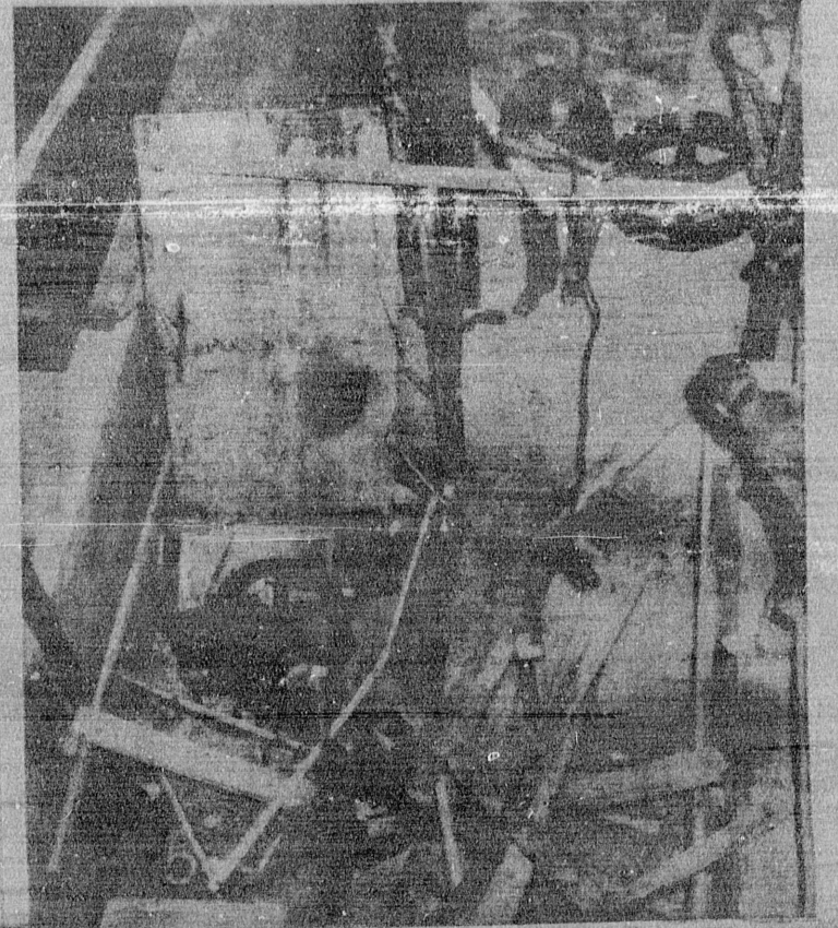
INSPECTING FALL SCENE . . . Workers and police investigators inspect the bottom of the elevator shaft where one man was killed and three others injured Friday when a temporary elevator tumbled 100 feet during construction at the Del Amo Shopping Center. (Herald Photo)
