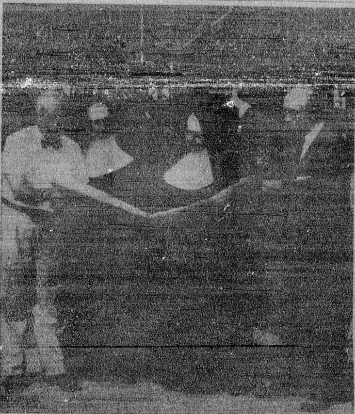
STUDY BLUEPRINTS . . . With third floor concrete poured in the construction of the Little Company of Mary hospital, Torrance Blvd. west of Hawthorne Blvd., a progress check was made last week by, left to right, George Leverenz, construction supervisor; Mother Lucy and Mother Virginia, both of the Little Company of Sisters of Mary; and Robert I. Plocoert Jr., president of the board. (Herald Photo)
