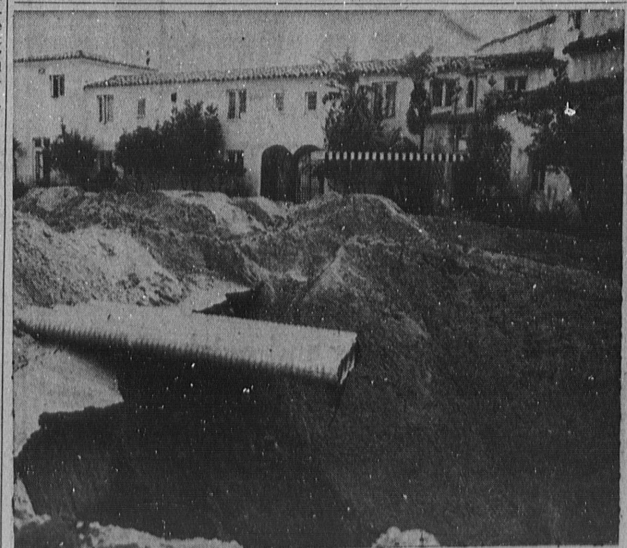
REPAIRS UNDER WAY . . . Repair work is still under way in many parts of the city following the heavy rains of 10 days ago. Here the gaping hole which nearly undermined the Riviera Beach Club is shown before the huge refilling task was completed. The club was threatened for some time during the height of the storm.
