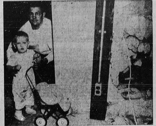
SURVEYING NARROW MISS . . . Fifteen-month-old Keith Hueth and his father, K. M. Hueth, of 2446 W. 174th St., survey the damage done to the Hueth garage Saturday evening when an automobile swerved out of control and crashed into the building. Keith was playing where is now standing when the crash occurred (additional accident photo with details was published in the Monday HERALD).
