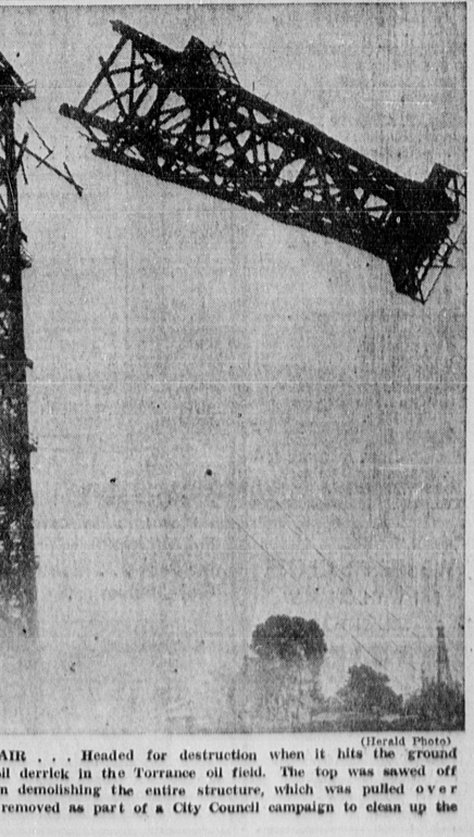
IT FLIES THROUGH THE AIR . . . Headed for destruction when it hits the ground is this 40-foot section of an oil derrick in the Torrance oil field. The top was sawed off Wednesday as the first step in demolishing the entire structure, which was pulled over later. The derricks are being removed as part of a City Council campaign to clean up the oil fields.
