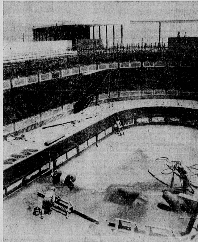
NEW HOME FOR FISH . . . This 600,000-gallon tank will house part of the fish in the Marineland of the Pacific. Visitors will be able to watch the fish from above, or from windows, placed in three different levels in the tank. The tank has been specially earthquake-proofed in construction.
