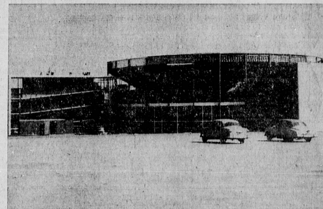
BEFORE . . . The partially completed Oceanarium, which is scheduled for completion by Aug. 28, will house some five to ten thousand fish. It will cost about $3,000,000.
