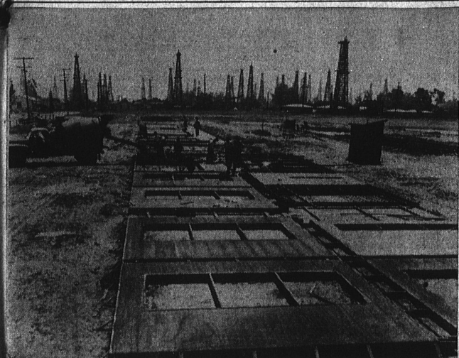
THESE ARE WALLS? . . . Although these workmen may appear to be pouring a concrete floor, they are actually pouring a cement wall for the new Howard E. Wood Elementary School. When hardened, sections will be hoisted into vertical position. Holes will be plugged with windows and doors. School has been delayed and may be delayed again by a shortage of cement.
