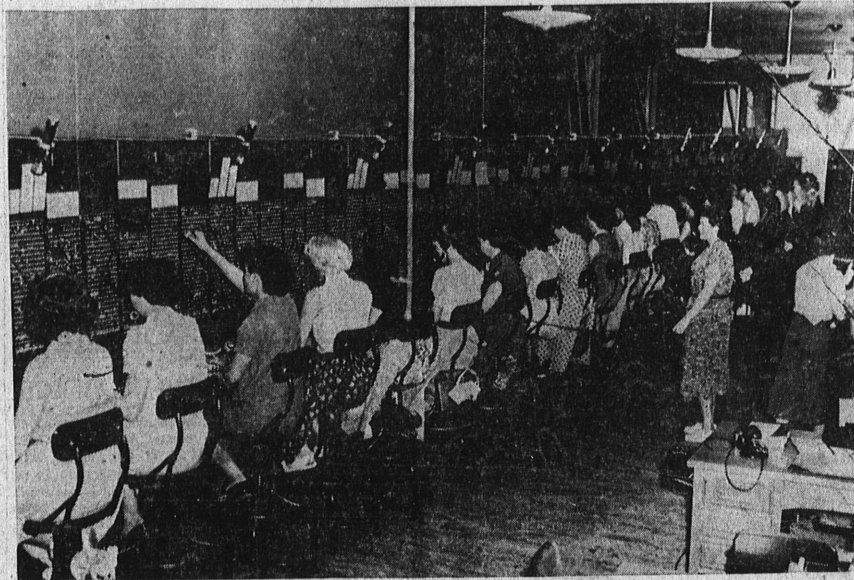
SOON A MEMORY . . . Activity such as that shown above will soon be a memory when Torrance telephone subscribers switch over to the long-awaited dial system on May 31. Pictured is the main telephone operator switchboard now in
