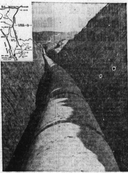
SOME OF THE MOST RUGGED COUNTRY IN THE SOUTHWEST IS TRAVERSED BY THE SAN DIEGO AQUEDUCT. The section here shown crosses the San Diego County-Riverside County line, continuing over the distant range. Water from the distant Colorado River will give San Diego and adjacent communities a supplemental supply with completion and dedication of a 71-mile Aqueduct Dec. 11. The conduit taps the Metropolitan Aqueduct in Riverside County. Dotted lines show extensions now under construction.
