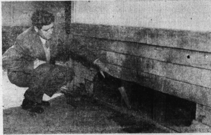
L. A. SCHOOLS RESTRAINED FROM REMOVING BUNGALOWS ... James L. Lynch, vice chairman of the Charter Committee and candidate for the Torrance Board of Education, points to the hole knocked in the siding of a bungalow at Torrance Elementary School preparatory to removal of the building by the Los Angeles school system to another location in the system. The Los Angeles schools have been restrained temporarily by court order from removal of Torrance school property pending a hearing on a permanent restraining order scheduled for March 19, in Superior court. City Judge John A. Shidler, taxpayer-plaintiff, alleged the property belongs to the taxpayers of Torrance under provisions of the education code. (Torrance Herald photo.)
