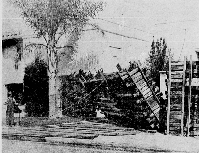
COMPLETING A CAMPAIGN . . . launched at the suggestion of the Torrance Herald on March 30, a city crew with tractor Wednesday tackled the barricades around the former Chamber of Commerce building, and the Herald photo above shows the first section falling to the ground to afford the Torrance residents and visitors a glimpse of the attractive structure. Crews are likewise removing the blackout shades from city lighting standards, and Torrance once more becomes a "well lighted" city. The removal comes out a promise by Mayor Tolson to the people and is the result of councilmanic action on May 9.
