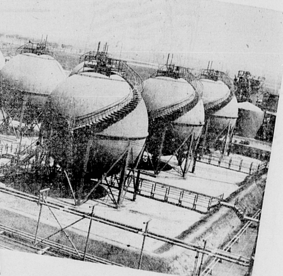
HUGE SPHEROID TANKS . . . are used for storing under pressure the many hydrocarbon streams in process at the Shell Chemical Division of Shell Union Oil Corporation at Torrance.
