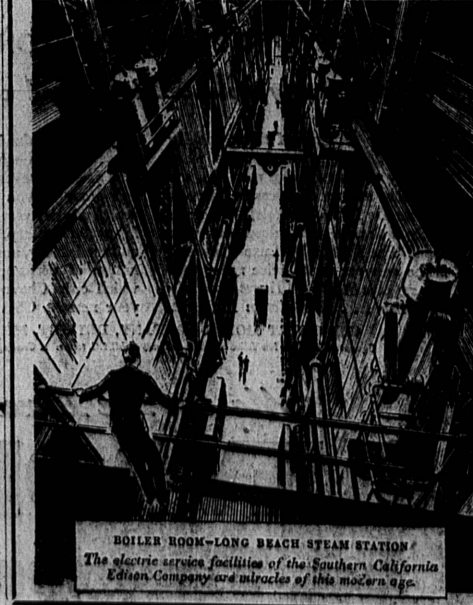
BOILER ROOM—LONG BEACH STEAM STATION The electric service facilities of the Southern California Edison Company are miracles of this modern age.
