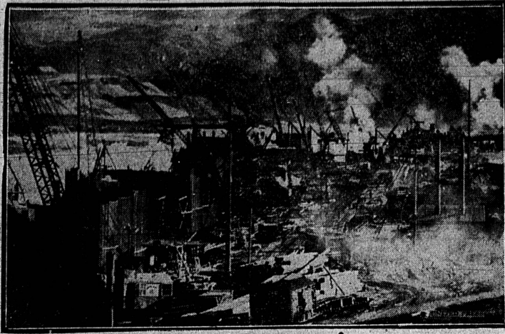
Grand Coule, on the Columbia river in central Washington, was a dusty desert place less than two years ago. Today it is a frenzied, roaring mass of cranes, power shovels and other machinery as 4,000 men rush work on the $63,000,000 federal power and irrigation dam project.
