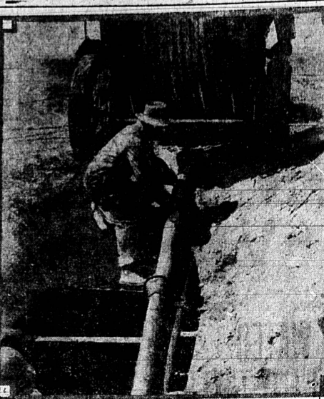
This shows how the Bell System placed more than 270 miles of its new $10,000,000 Los Angeles-San Francisco cable underground in fibre conduit. The entire cable is 415 miles long, and weighs 18,000,000 pounds.
